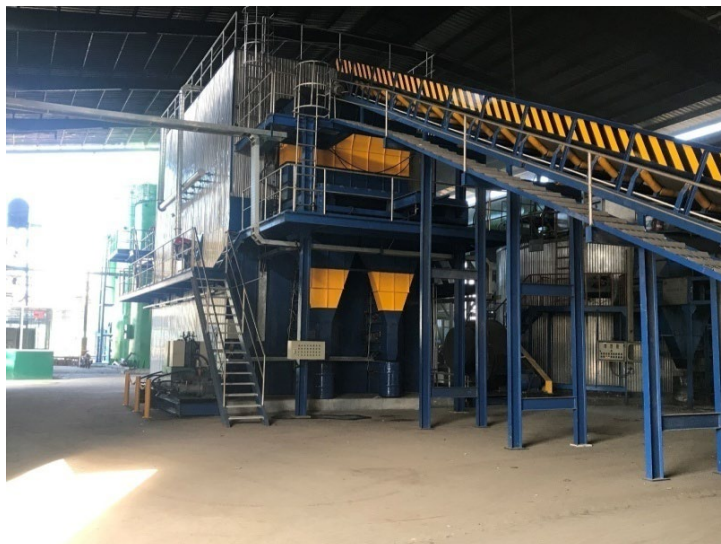
Figure 13 Waste incinerator in 2021 (Source: Hoai Le, evaluation tam)
