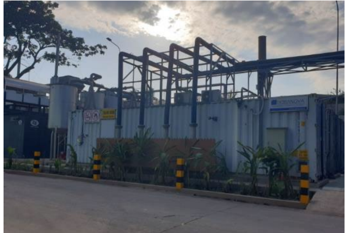
Figure 16 Landfill gas collection system in Dec 2021 (Source: Hoai Le, evaluation team)
