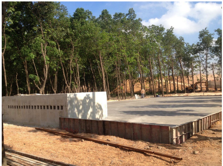
Figure 6 Foundations for the gas pump and generator area in 2018 (Source: Doranova Oy)
