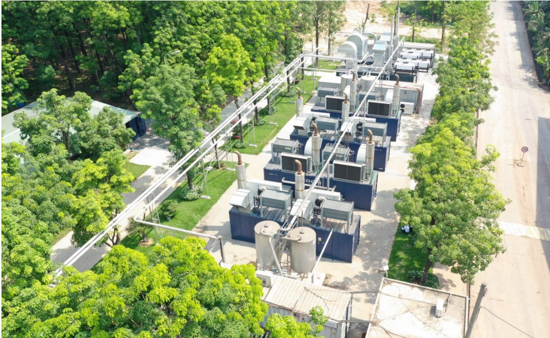
Figure 12 The CHP units and related infrastructure in 2021. In the front are the filters installed during the CCS project. The blue containers are the CCS project installed capacity of 1 600 kW and the black containers in the back the additional 720kW implemented in the EEP financed project. (Source: Hoai Le, evaluation team)
