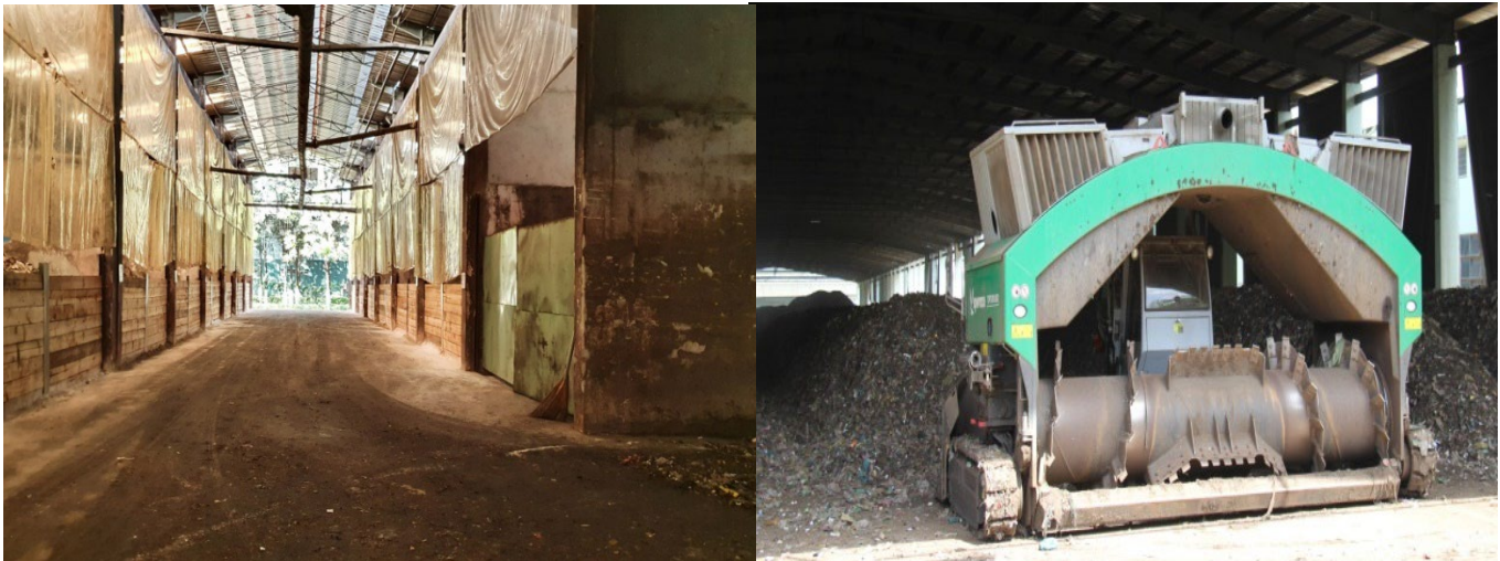
Figure 15 Composting tanks and maturing stage (Source: Hoai Le, evaluation team)
