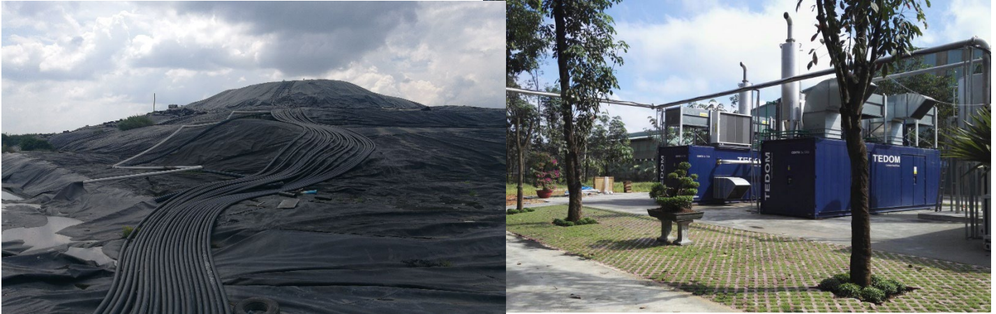
Figure 7 Covered landfill with the gas transfer lines and the installed CHP units. (Source: Doranova Oy)
